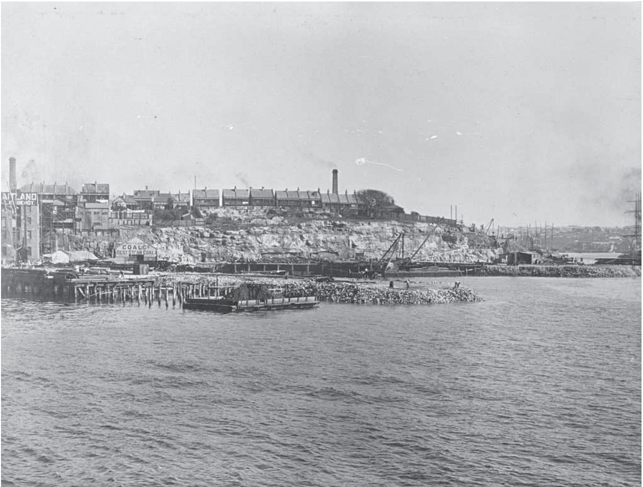
Figure 5.5.6: Anon, 1917, Wharf construction, Jones Bay, about 1917 (ML Government Printing Office GPO 1_47213/digital order no. d1_47213)
