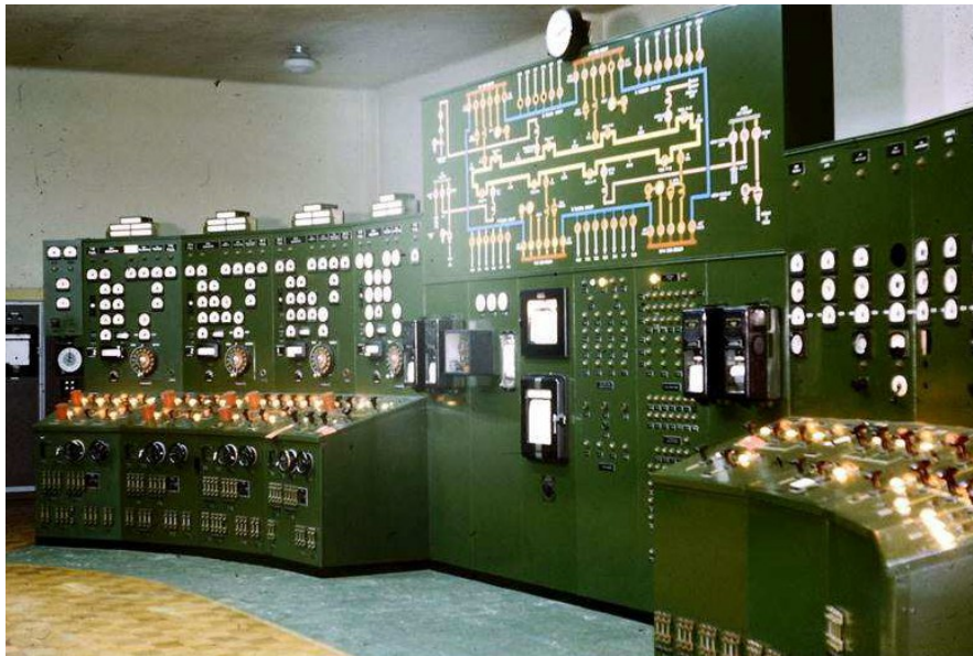
Pymont 'B' Power Station. Electrical Control Room including the Grid Control Centre. On the panel at left are controls for the four 50 MW turbo-alternators.
